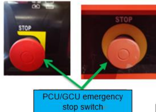
Fig. 9.7 Emergency stop switches of PCU and GCU
